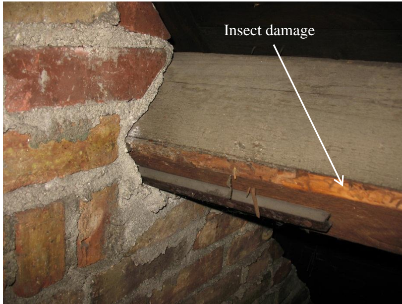
Figure 4. Insect damage visible on corner of purlin near bearing at east wall of sanctuary; not structurally significant.
