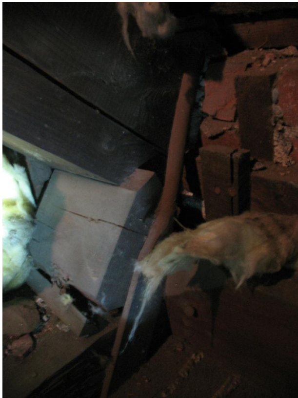
Figure 6. Typical truss bearing at exterior masonry wall (at buttress). Actual bearing condition concealed by masonry beyond steel connection tie in foreground.
