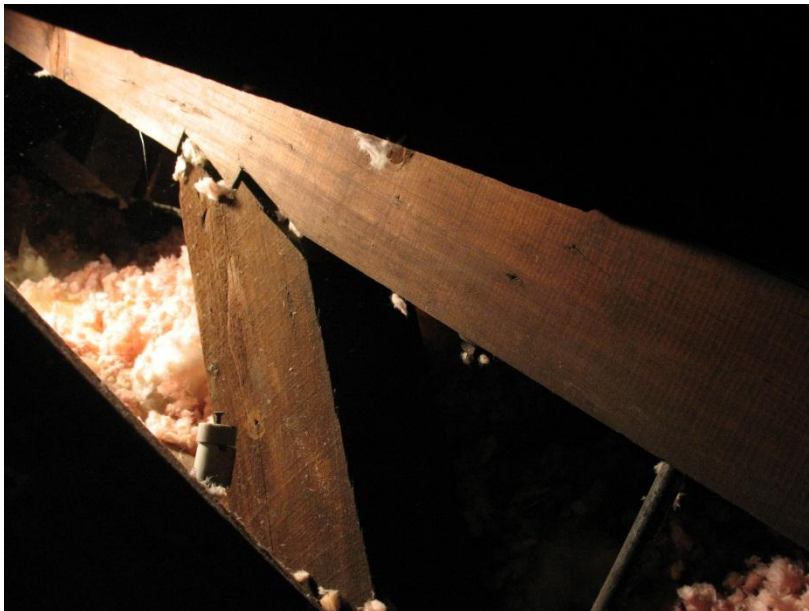
Figure 8. Example of disengaged compression web member connection (double bird's mouth) on typical main truss consistent with downward displacement of the arch and spreading of the top chords.
