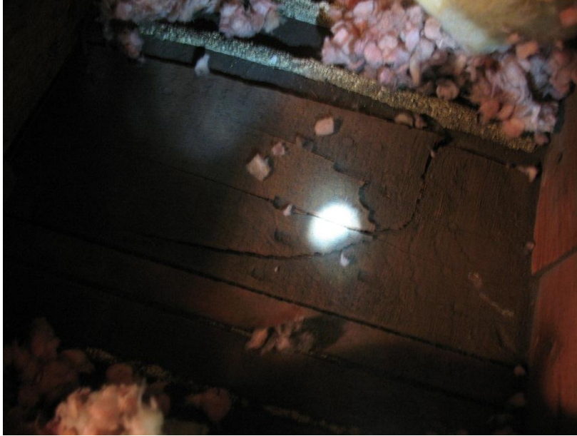
Figure 7. Partial fracture of built-up main arch member of barrel vault in typical truss.
