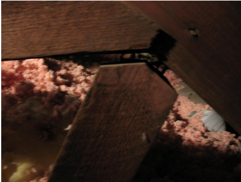
Figure 9. Another example of a typical truss compression strut with toe-nailed connection partially pulled-out.
