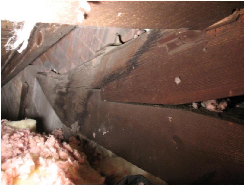
Figure 5. South bearing of choir loft truss on interior masonry wall. Note moisture staining; no deterioration observed.
