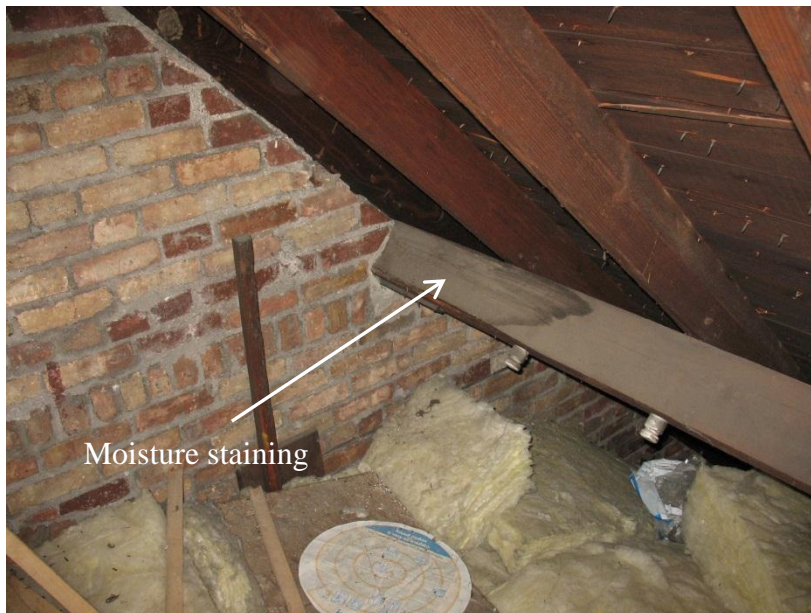
Figure 4a. Another view of the purlin bearing at east wall of sanctuary showing extent of moisture related staining. No significant wood decay was observed.
