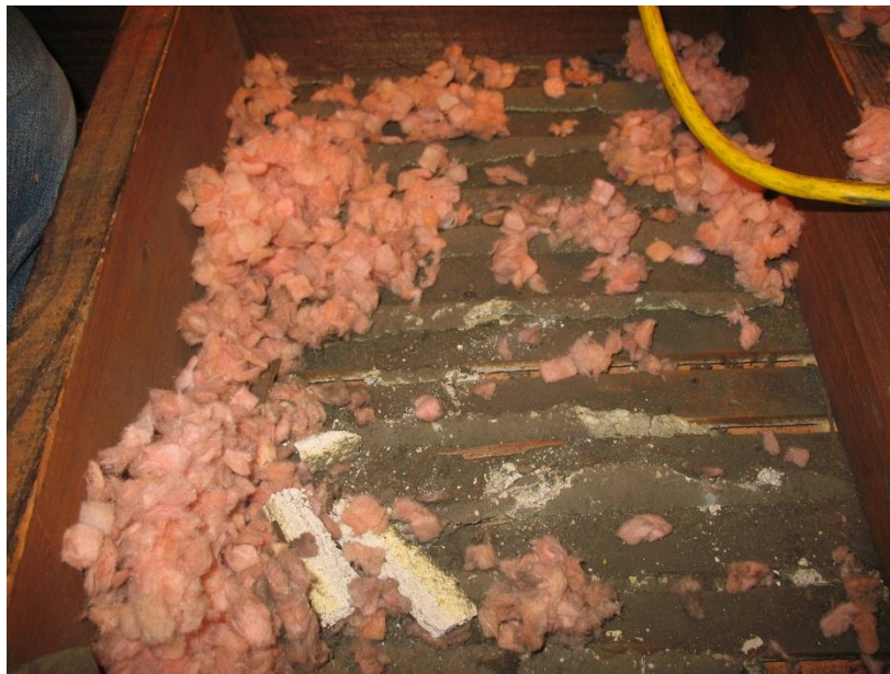
Figure 3. Original lath and plaster largely intact beneath insulation; plywood infill appears to have been installed over top of existing plaster.
