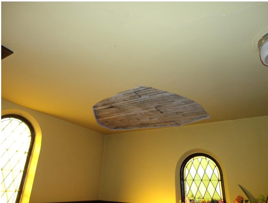
Figure 43. Plaster ceiling failure in southeast sacristy.
