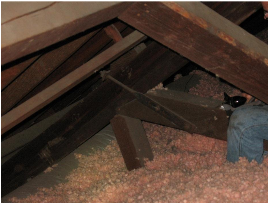
Figure 31. Steel tie rod connecting strut to top chord further down typical truss.
