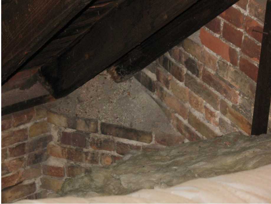
Figure 32. Rafters bearing on wood sill on top of masonry wall near southwest corner. Note light discoloration near bearing location of rafters as possible moisture-related deterioration.
