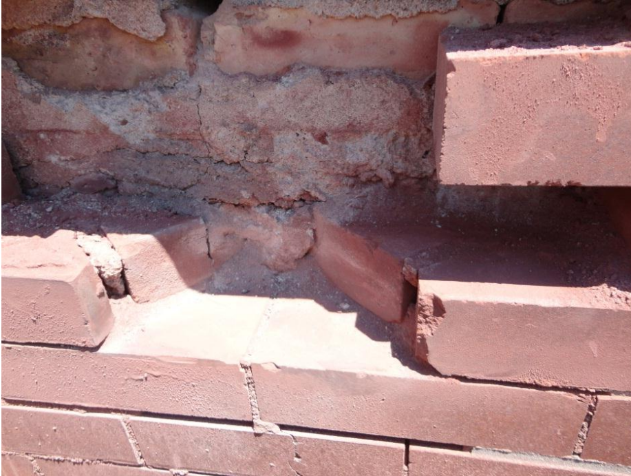
Figure 7. Notch-cut brick construction, as observed in the inspection opening on the east elevation of the lower bell tower.
