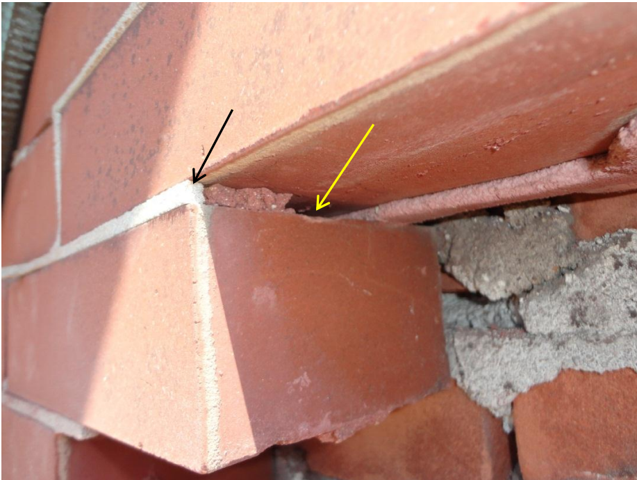
Figure 8. South elevation gable inspection opening showing the middle void between the original veneer mortar joints (yellow arrow), along with the lighter colored skim repointing failing near the opening (black arrow).
