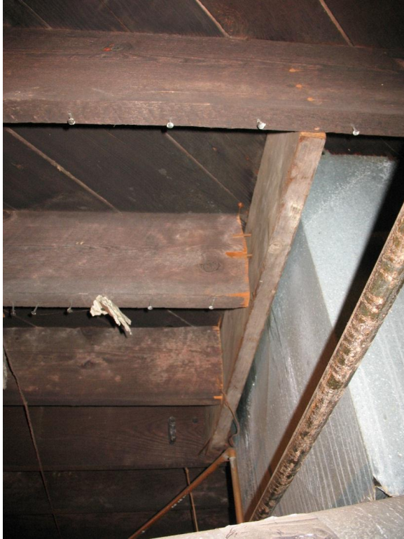
Figure 28. End nailed joist connections to frame around a ductwork penetration of the floor deck. These should be supplemented with steel joist hangers.
