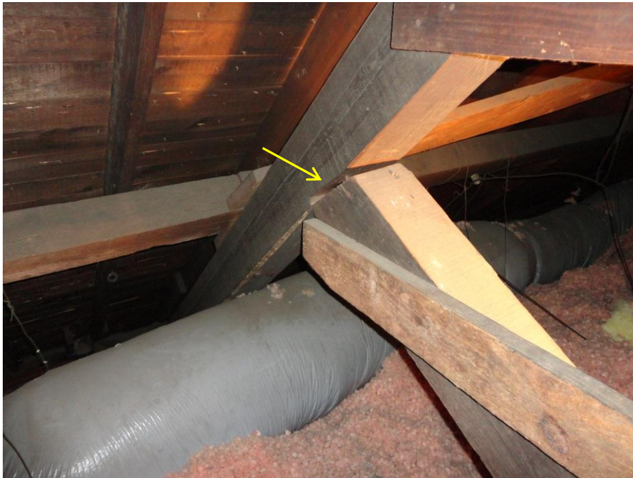
Figure 33. Partial view of north side of first truss from the west wall. Note bottom chord extension nailed to top chord has separated (arrow).
