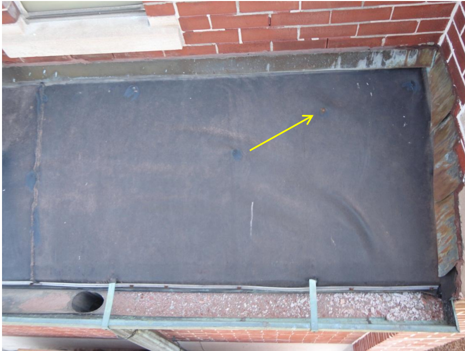
Figure 15. Nail penetrating lower roof EPDM membrane (arrow) on south elevation near bell tower. Note also bulging of membrane and masonry debris in gutter away from downspout.
