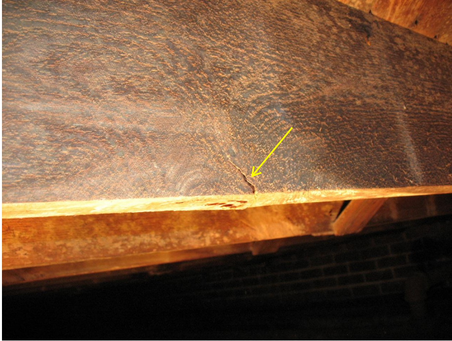
Figure 26. Partial fracture of 2x10 floor joist originating from knot on bottom of member.
