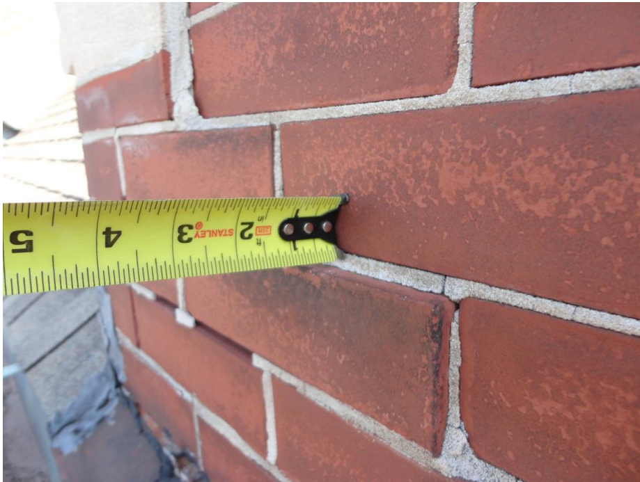
Figure 10. Veneer brick displaced approximately 1/4 inch outward on south elevation middle gable.
