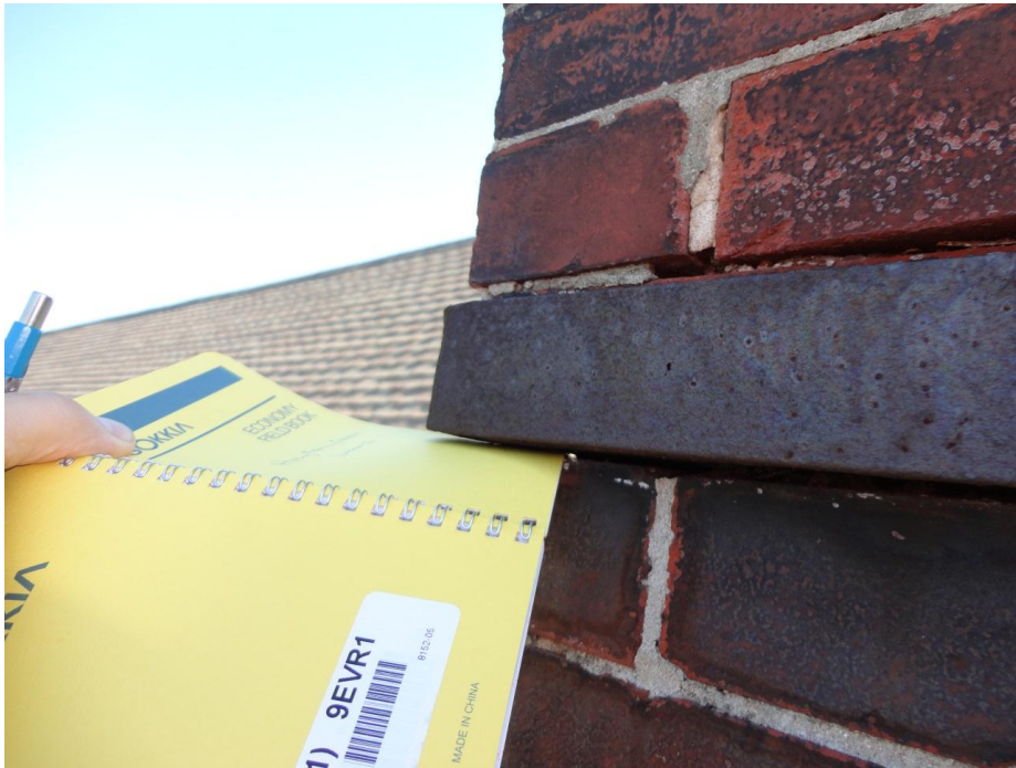
Figure 18. Severe deterioration of chimney mortar joints in vicinity of steel band. Some joints completely missing.
