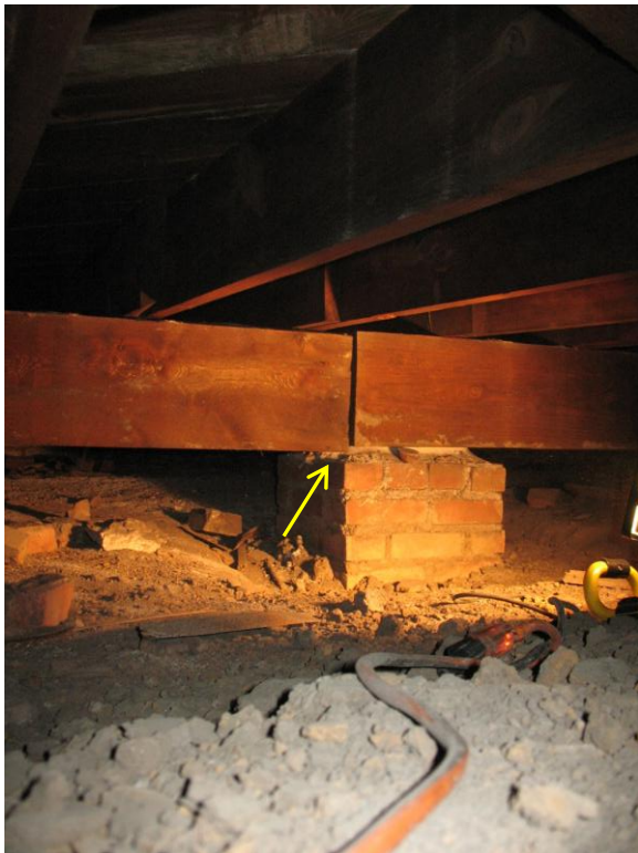
Figure 25. Near 2x12 member of built-up main floor beam does not bear on masonry pier (arrow). Other 2x12 members do bear on pier.
