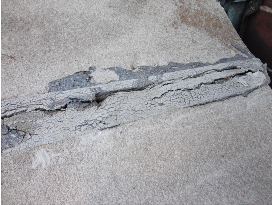
Figure 13. Failed sealant along joint in limestone coping on west main gable showing patterned cracking induced by ultra-violet exposure.
