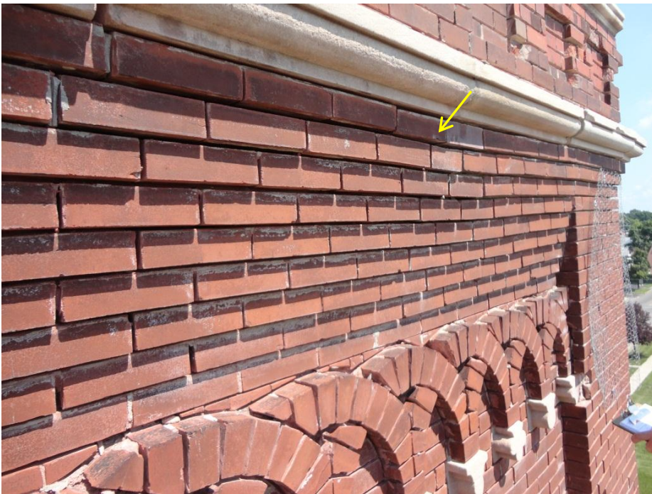
Figure 21. Visible downward displacement (arrow) of recessed courses above main arches on upper bell tower.
