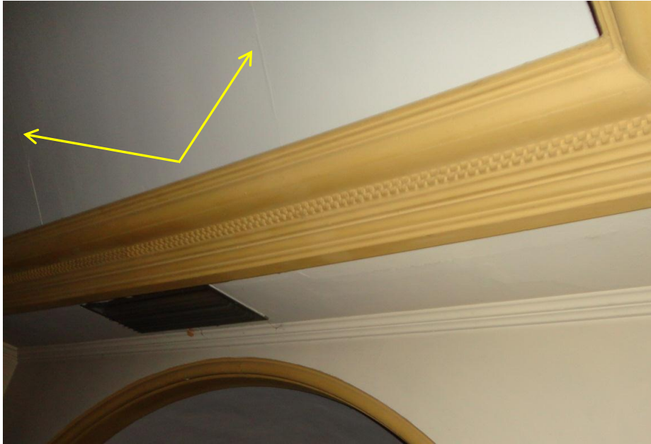
Figure 40. Parallel cracking in plaster skim over plywood panels at barrel vault.
