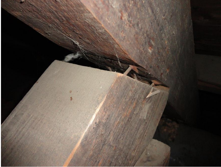
Figure 36. Partial pull-out of westernmost truss bottom chord extensions at connection to top chord. Separation likely old given dark coloration.
