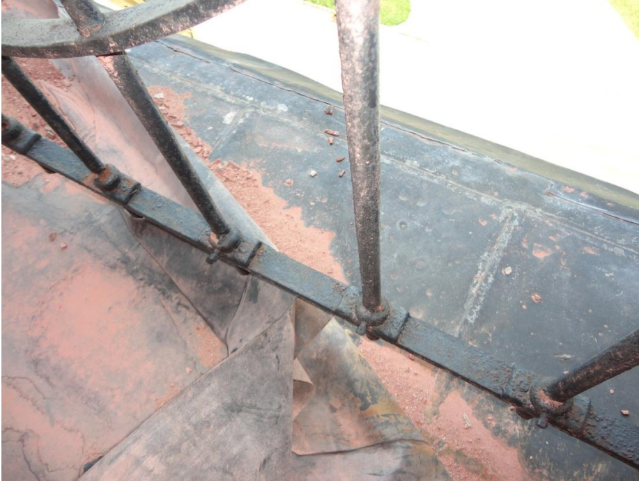
Figure 22. Belfry membrane failed and peeling back from roof edge; underlying original lead-coated copper intact.
