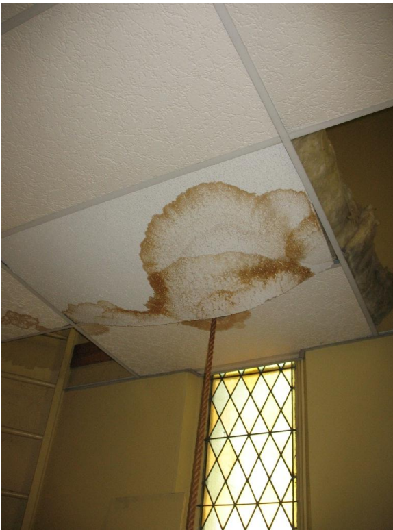
Figure 23. Water damage on drop ceiling of bell tower interior. Note belfry rope hanging through gap in the ceiling.
