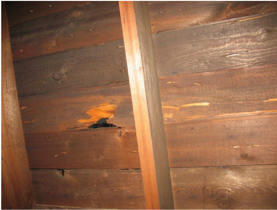
Figure 38. Typical damage to roof decking.
