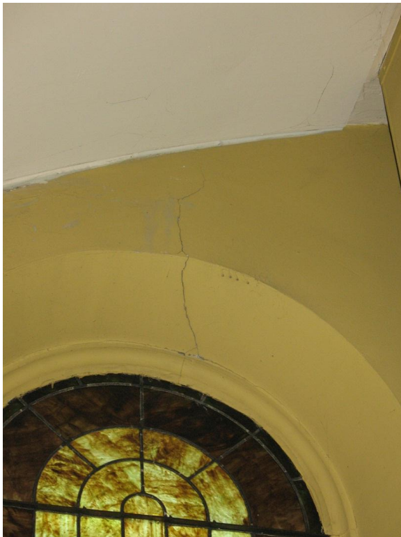
Figure 41. Crack in plaster at south window of west main gable.
