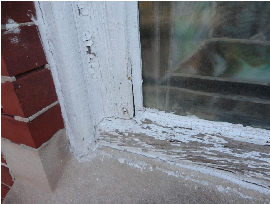
Figure 14. Peeling and missing paint coating at wood window framing.
