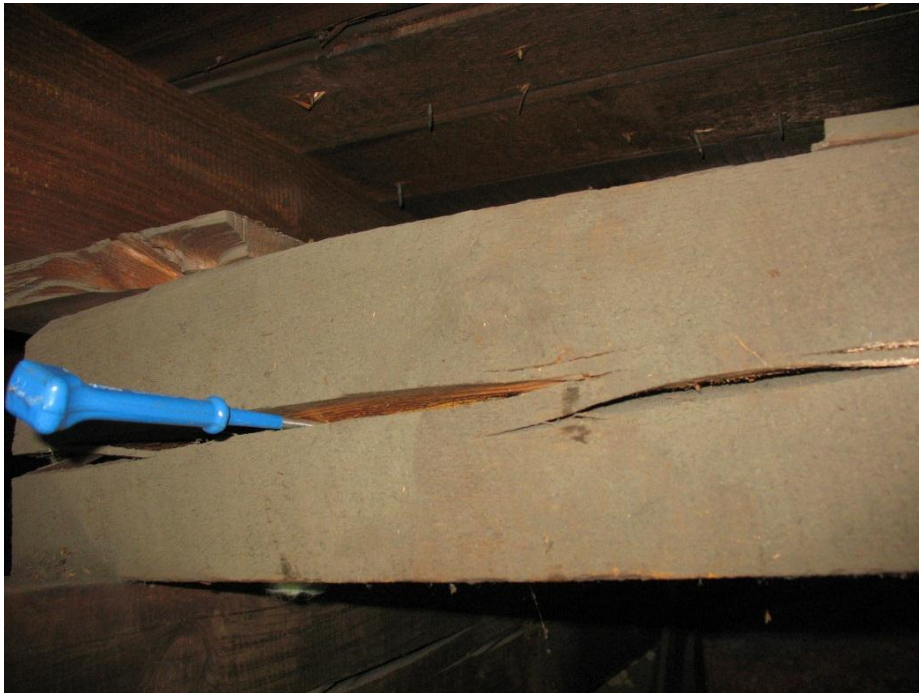
Figure 37. Checking of purlin, approximately 2.5 inches deep. Light coloration within crack may indicate recent formation or growth of this check.
