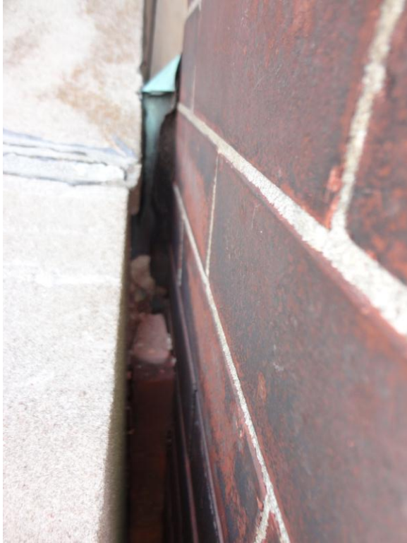
Figure 9. Inappropriate/missing flashing at interface of bell tower and south end of west main gable. Water can freely penetrate into the building here from the gable roof and direct exposure from above.
