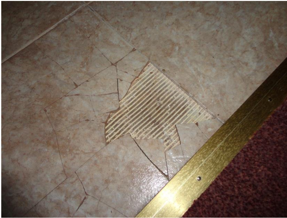
Figure 42. Cracked flooring tile near the information table.
