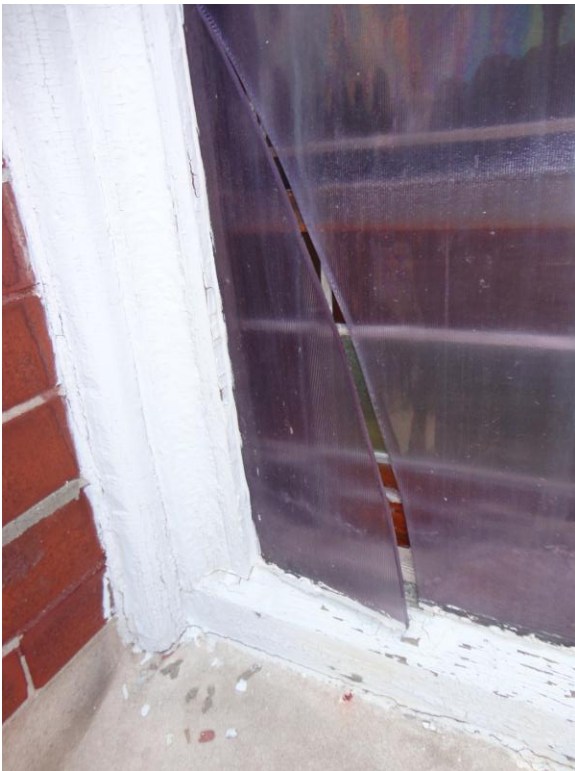
Figure 12. Broken protective glazing at main stained glass window on west face of bell tower.
