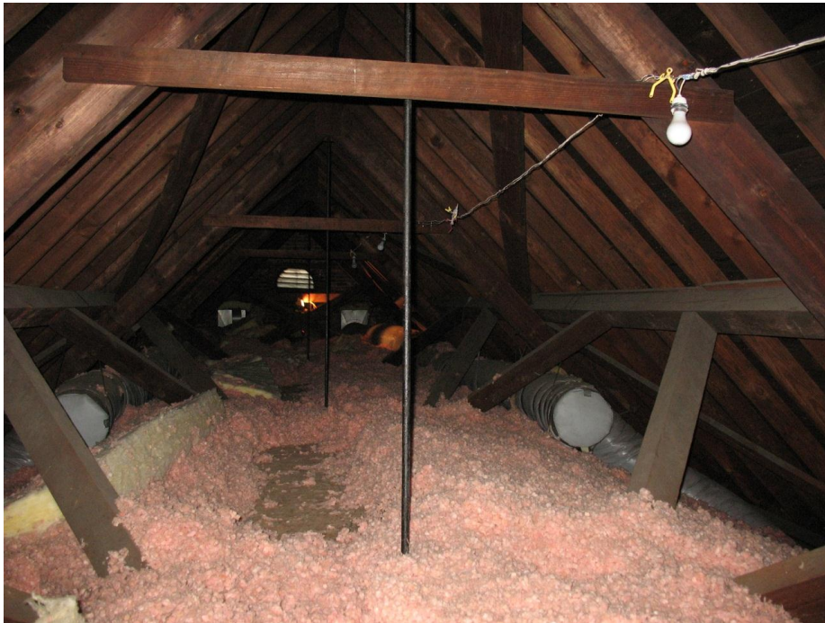
Figure 29. Roof framing viewed from center of attic looking west. Dark vertical bars are steel tension rods at center of each typical truss.
